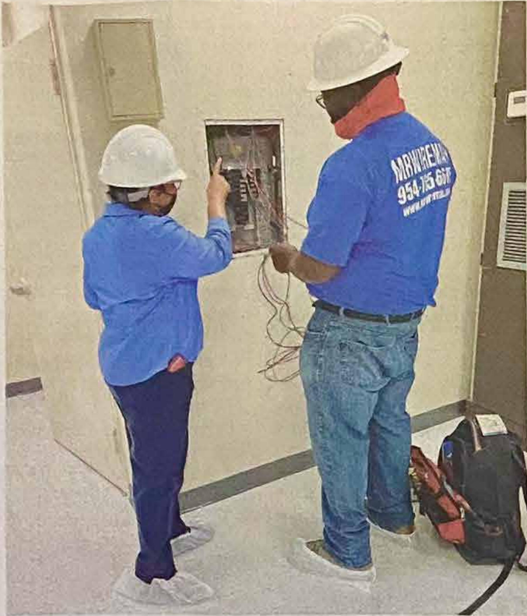
Margaret Anglin (L) working on a project installing a computer lab in West Palm Beach. COURTESY OF MARGARET ANGLIN
